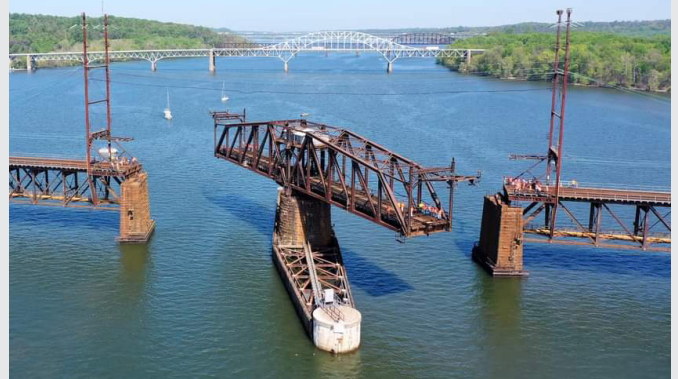
The existing bridge was built in 1906 and is nearing the end of its useful life. The aging infrastructure creates speed and capacity constraints, operational inflexibility, maintenance difficulties, and conflicts with marine traffic.
