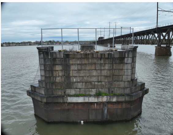
Bird deterrent netting was installed on the remnant 1866 piers in February 2024 to prevent pre-demolition nesting.
