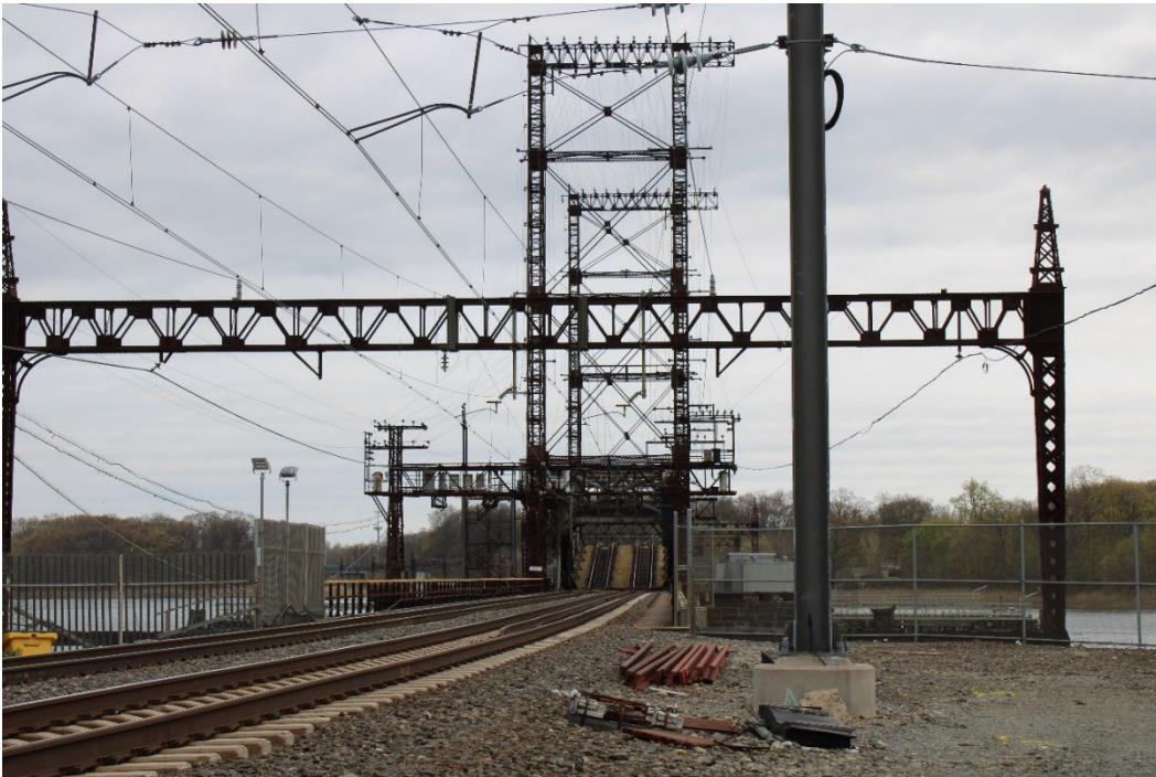
Photograph 5. View of Amtrak Pelham Bay Bridge with movable center span open looking northeast (4/25/22)
