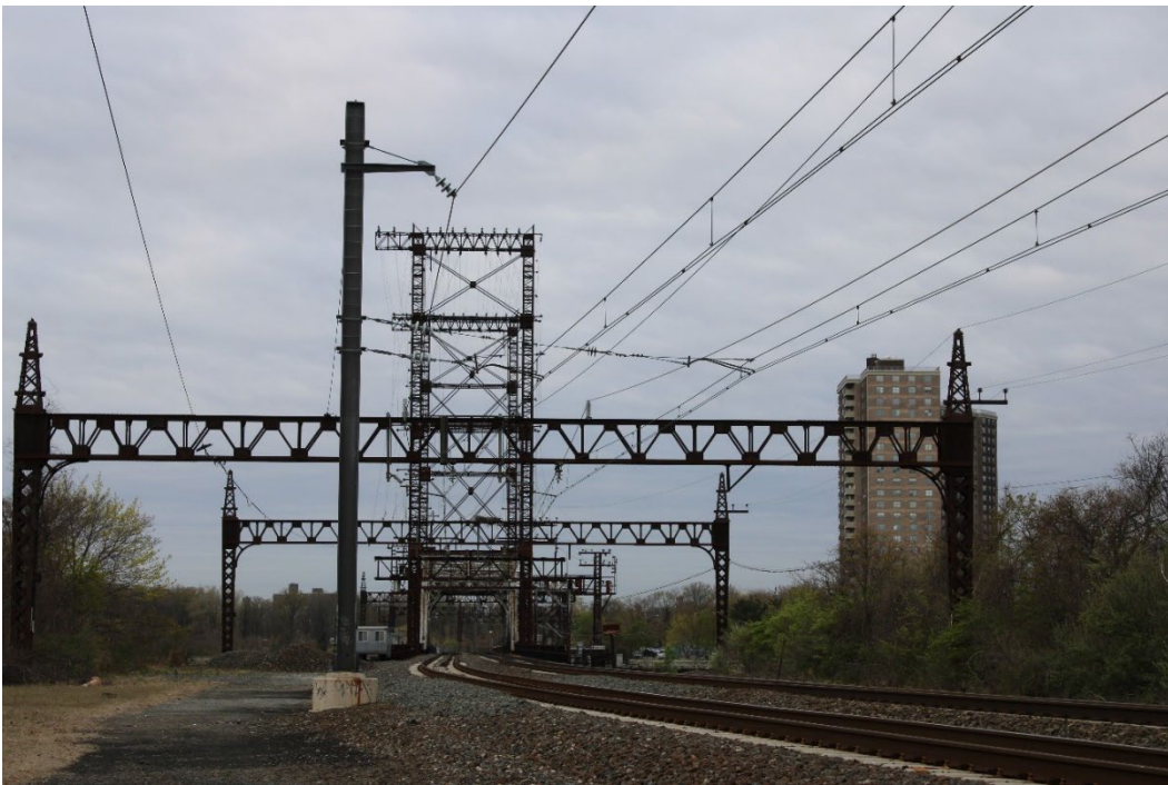
Photograph 4. View of Amtrak Pelham Bay Bridge looking southwest (Co-op City in the background) (4/25/22)
