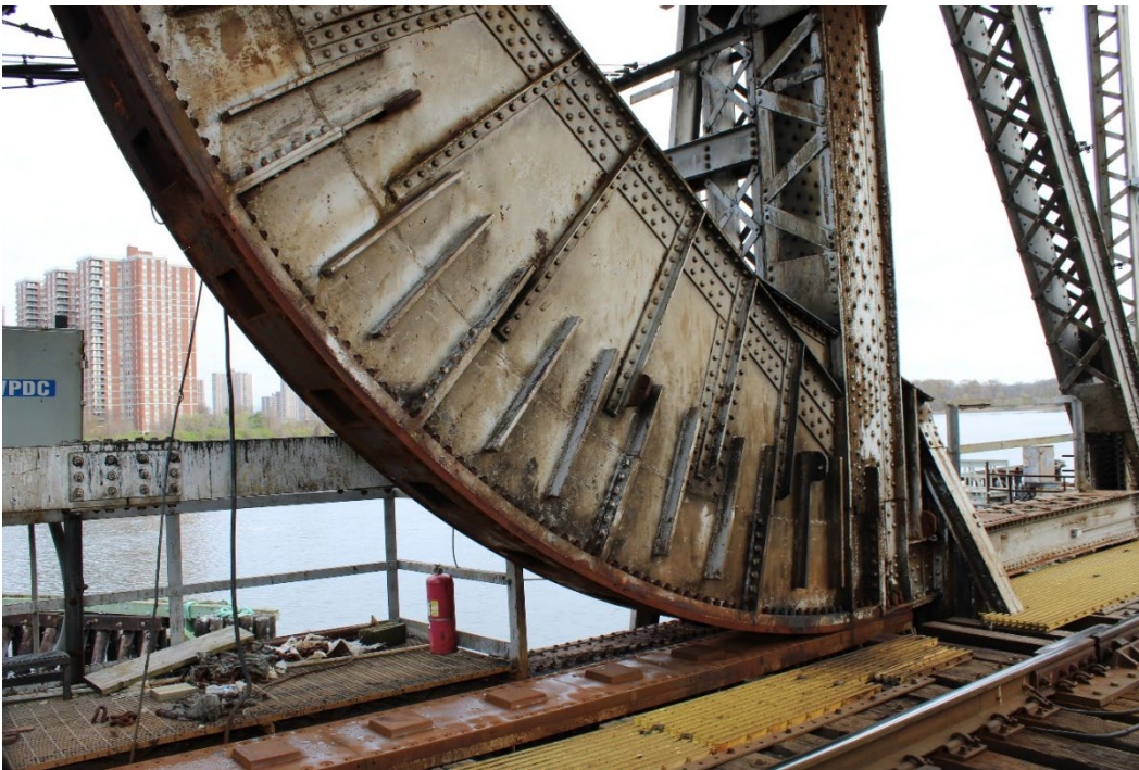
Photograph 6. View of Scherzer Rolling Lift component of Amtrak Pelham Bay Bridge looking north (4/25/22)
