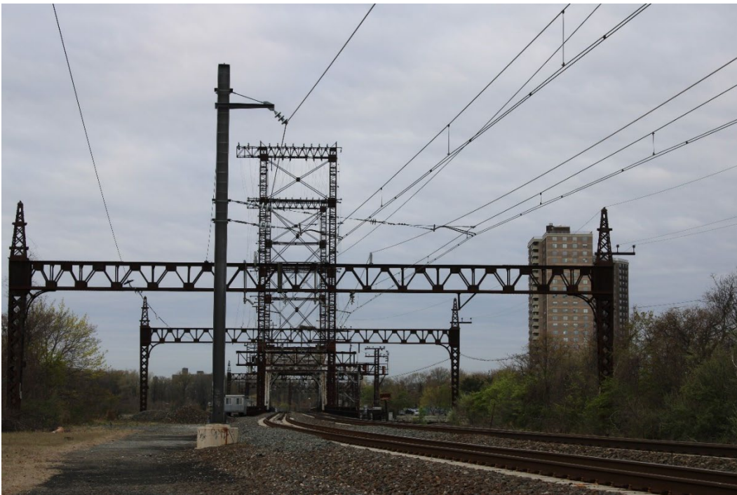
Photograph 4. View of Amtrak Pelham Bay Bridge looking southwest (Co-op City in the background) (4/25/22)
