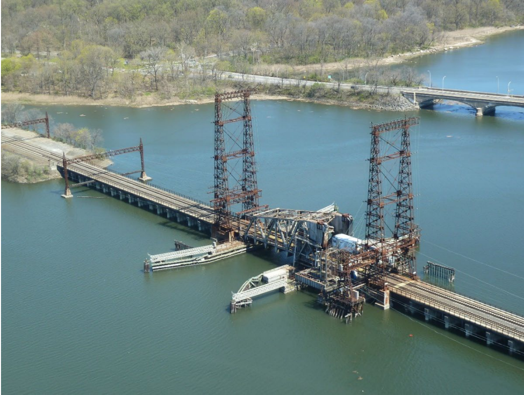
Photograph 1. View of Amtrak Pelham Bay Bridge looking east (Shore Road Bridge in the background) (4/20/22)
