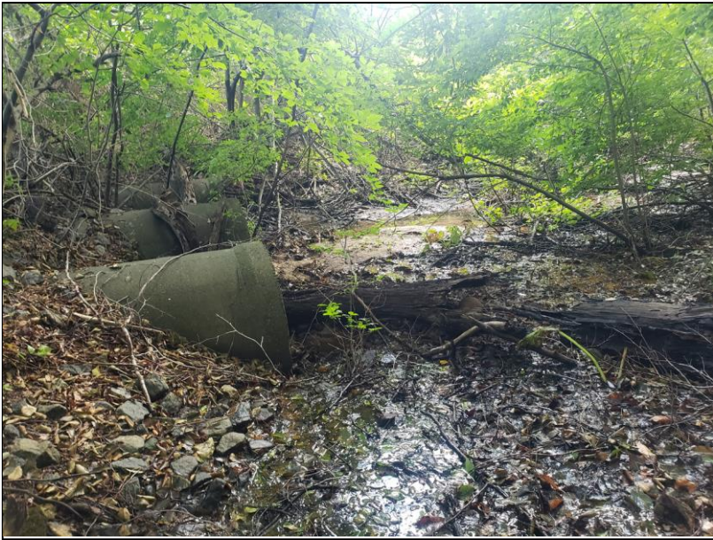
Photo 13: Wetland '200'; Ragged Rock Brook culverts under access roadway to earth products recycling facility; facing northwesterly
