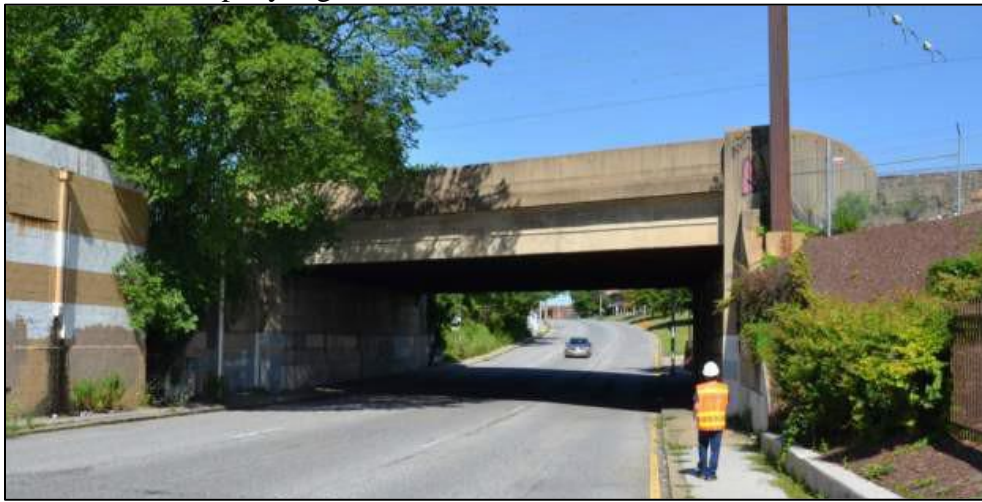
Plate 5: View looking northwest at the bridge carrying the B&P / Philadelphia, Baltimore and Washington Railroad over West Mulberry Street.
