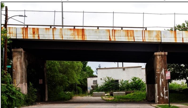
Plate 25: View looking north at the bridge carrying West Lafayette Avenue over the rail line, showing the approximate location of the new alignment. The bridge superstructure and piers will be rebuilt and reconfigured in this area, and the grade beneath the bridge lowered over 30 feet.
