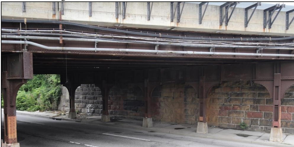
Plate 9: View looking north underneath the West Franklin Street bridge showing the stone abutment, riveted steel support columns, and the concrete from the 1990s deck replacement.
