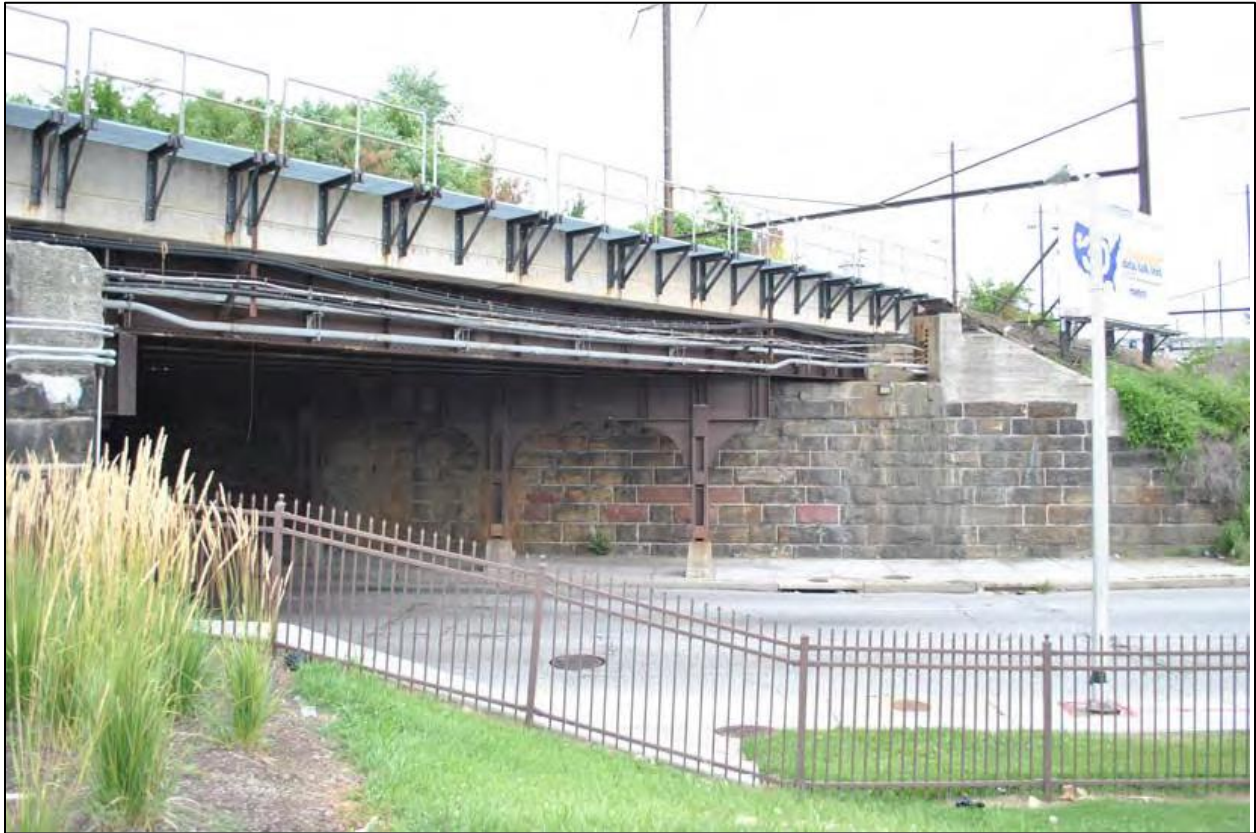
Plate 22: View looking north at the bridge over West Franklin Street, showing the stone abutment and wingwalls. The new bridge will be located to the west, which is to the left in this photo.
