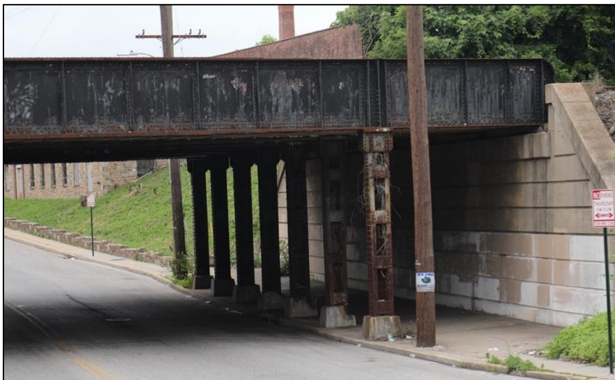
Plate 2: View looking northwest underneath the North Franklinton Road bridge showing the abutment, in-line wingwalls, and steel columns.
