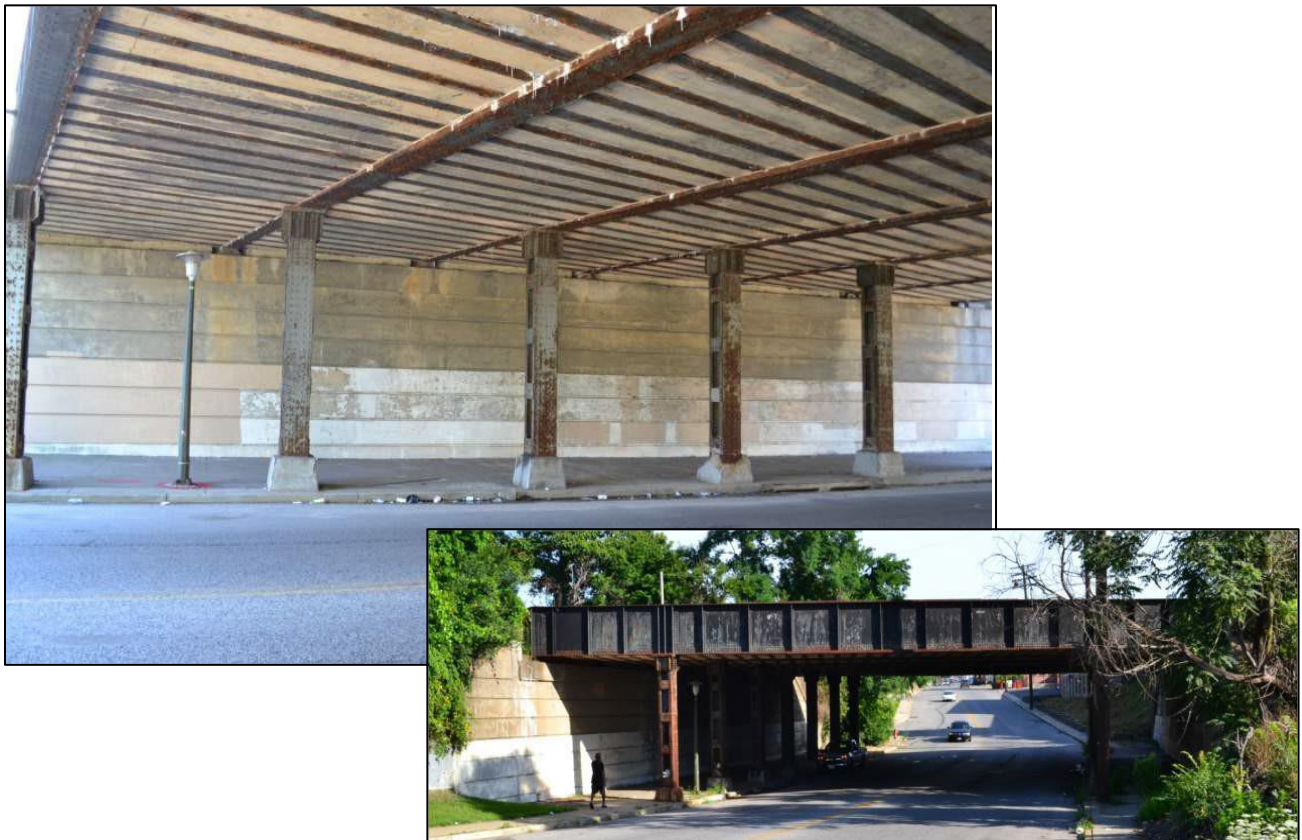
Plate 19: The bridge over North Franklinton Road, showing the underside of the bridge with the steel girders supported by riveted steel columns and the concrete abutments. All steel elements shown will be removed, and the concrete abutments and wingwalls will be modified.
