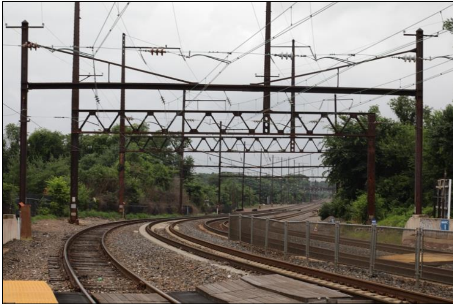
Plate 35: View of existing power lines looking west from the West Baltimore MARC Station, showing catenary and transmission poles.
