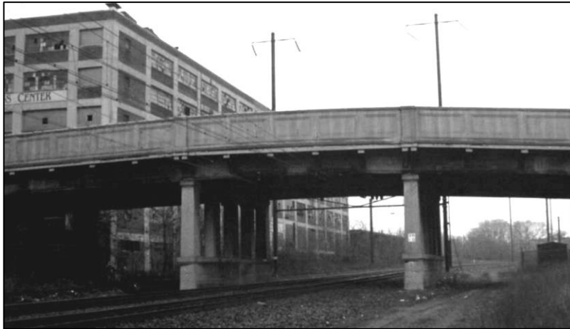
Plate 10: January 1995 view looking north at the bridge carrying West Lafayette Avenue over the B&P / Philadelphia, Baltimore and Washington Railroad. Tim Schoen, Maryland State Highway Administration, photographer.
