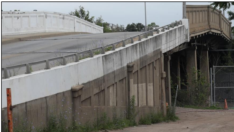
Plate 11: View looking east at the Classical detailing on the bridge carrying West Lafayette Avenue over the B&P / Philadelphia, Baltimore and Washington Railroad.
