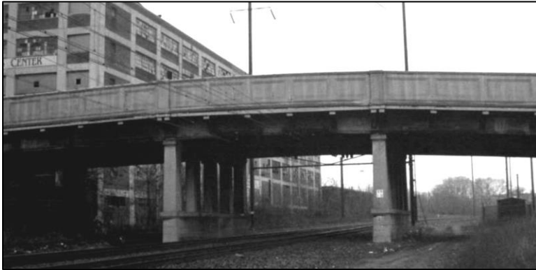
Plate 24: January 1995 view looking north at the bridge carrying West Lafayette Avenue over the B&P / Philadelphia, Baltimore and Washington Railroad. Tim Schoen, Maryland State Highway Administration, photographer. This central portion of the bridge, which is the only portion with Classical detailing, will not be altered.
