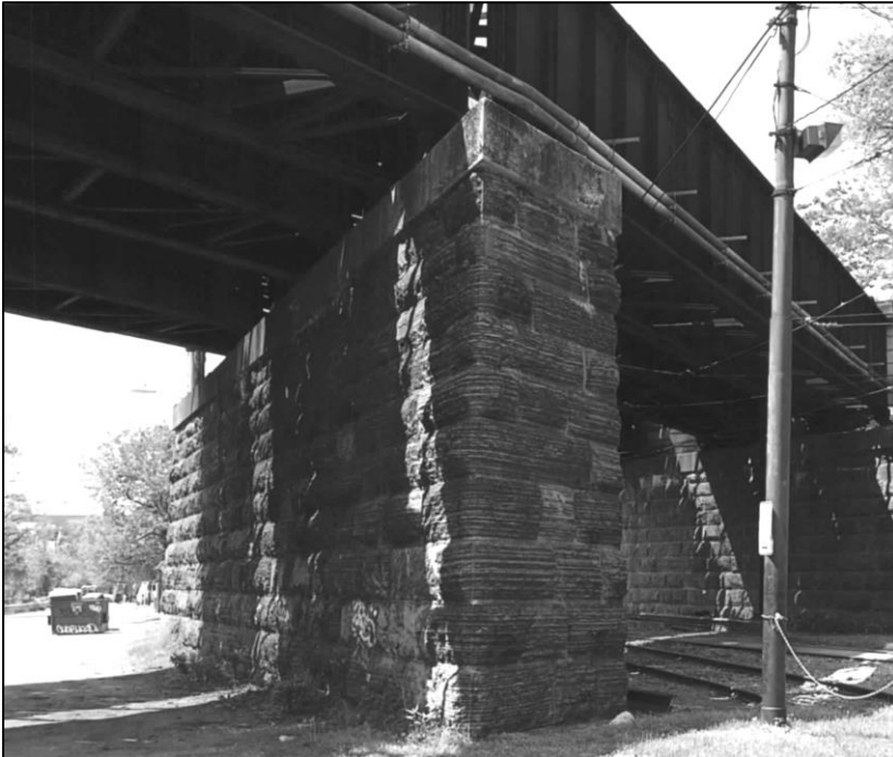
Plate 27: The B&O Railroad, Baltimore Belt Line Bridge over Jones Falls Valley, showing the stone pier that needs to be altered to allow for the new alignment.
