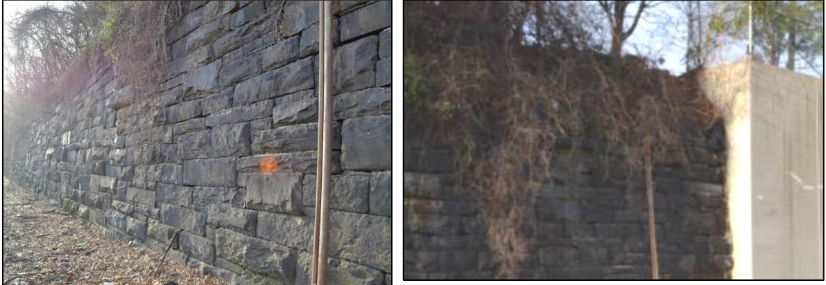
Plate 30: Retaining wall (left) between the B&O Railroad, Baltimore Belt Line Bridge and the light rail, and the transition area (right) between the stone wall and the concrete wall.
