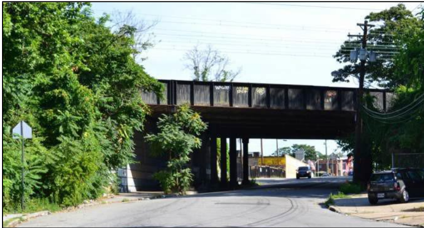
Plate 3: View looking south at the bridge carrying the B&P / Philadelphia, Baltimore and Washington Railroad over North Warwick Avenue.
