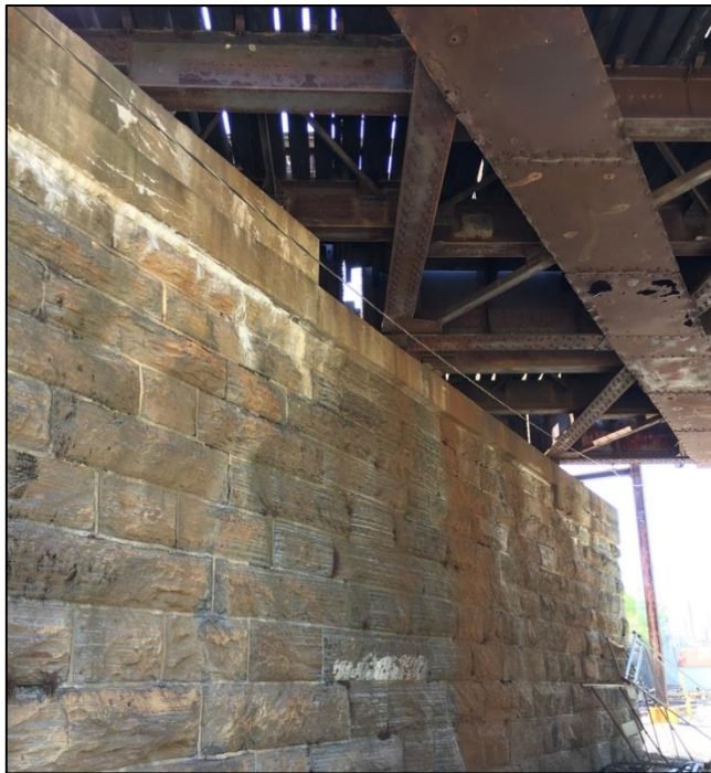
Plate 14: Limestone pier of the B&O Railroad, Baltimore Belt Line Bridge over Jones Falls Valley.
