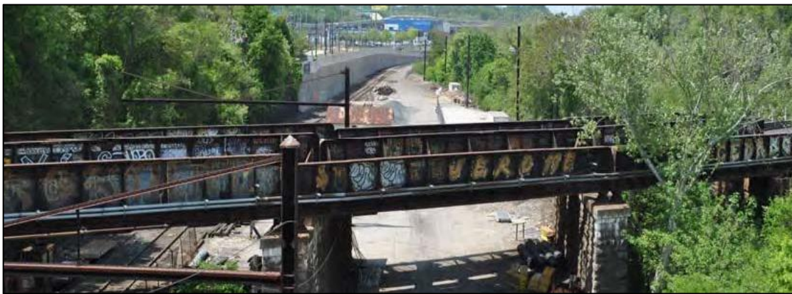
Plate 31: View looking northwest at the B&O Railroad, Baltimore Belt Line Bridge. The concrete retaining wall of the light rail in the upper left of the photograph meets the stone retaining wall, which in this photo is concealed behind the trees and bridge.
