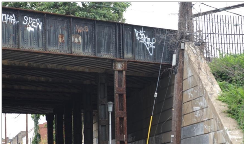
Plate 4: View looking northeast underneath the North Warwick Avenue bridge showing abutment, in-line wingwalls, and steel columns.
