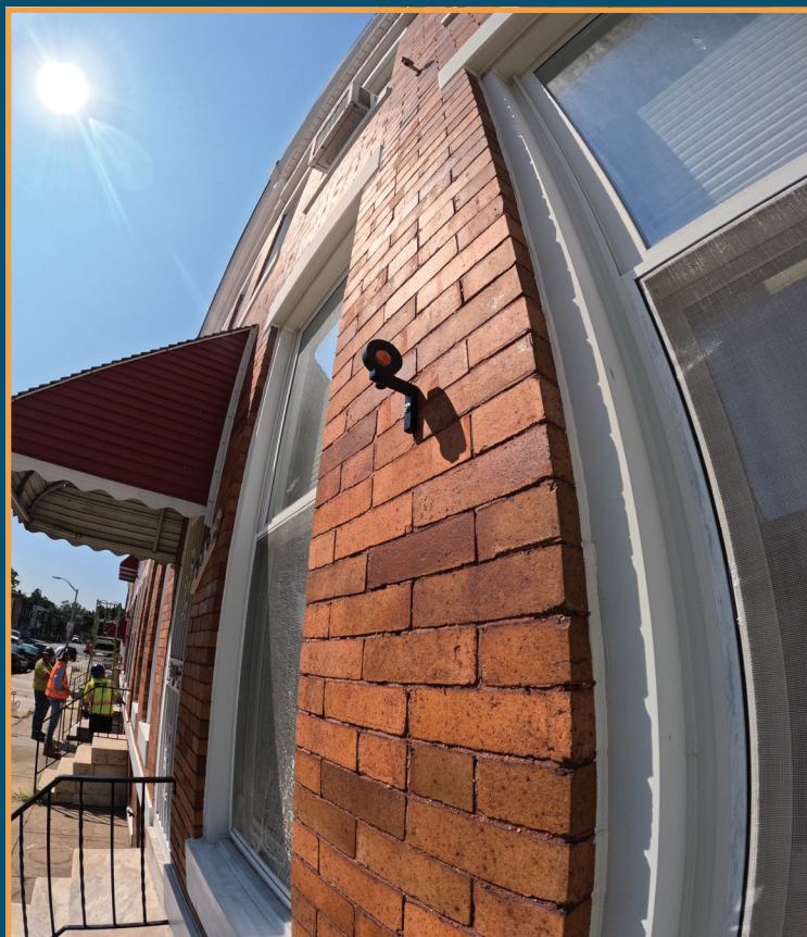
Installed tilt monitor
